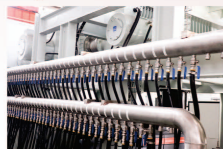
Cooling Water Manifold
